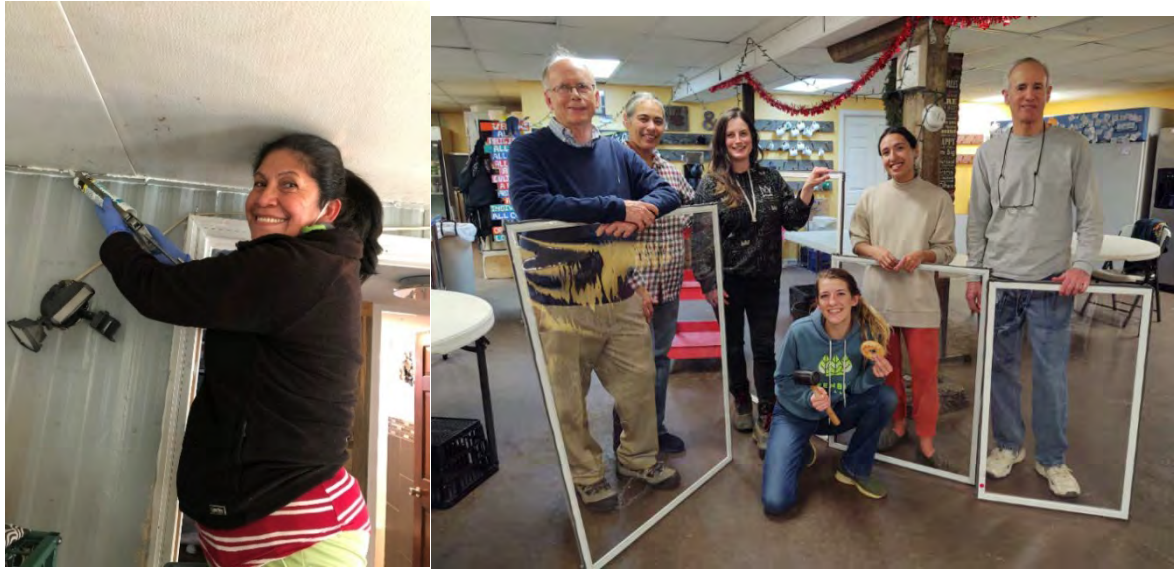
Energy Savers Network doing weatherization of low-income homes (Left) and creating custom storm windows (right)
