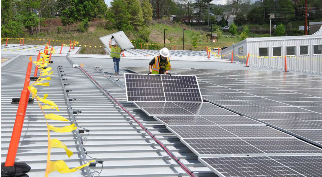
Solar Installation at Isaac Dickson School
